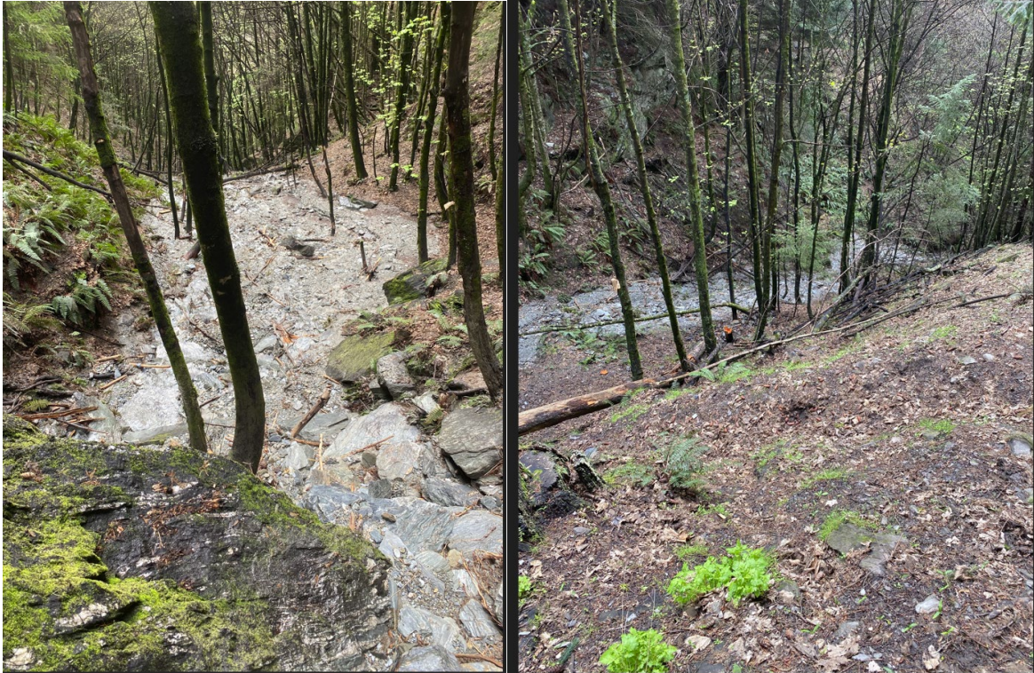
Photographs 9 and 10. Debris in Area 2 – Reavers Creek.
