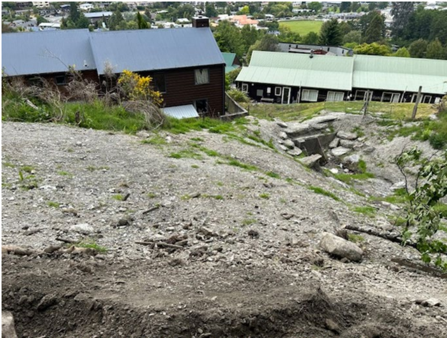
Photograph 3. Reavers Creek and the stormwater culvert and debris grate. Source - Sean Dent 27.11.23.
