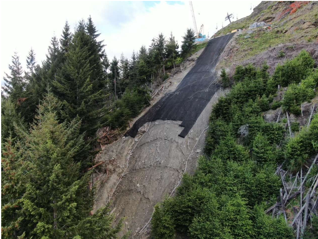
Figure 1.1: Showing a bulb of uncontrolled debris fill material in the upper Reavers Creek catchment.
