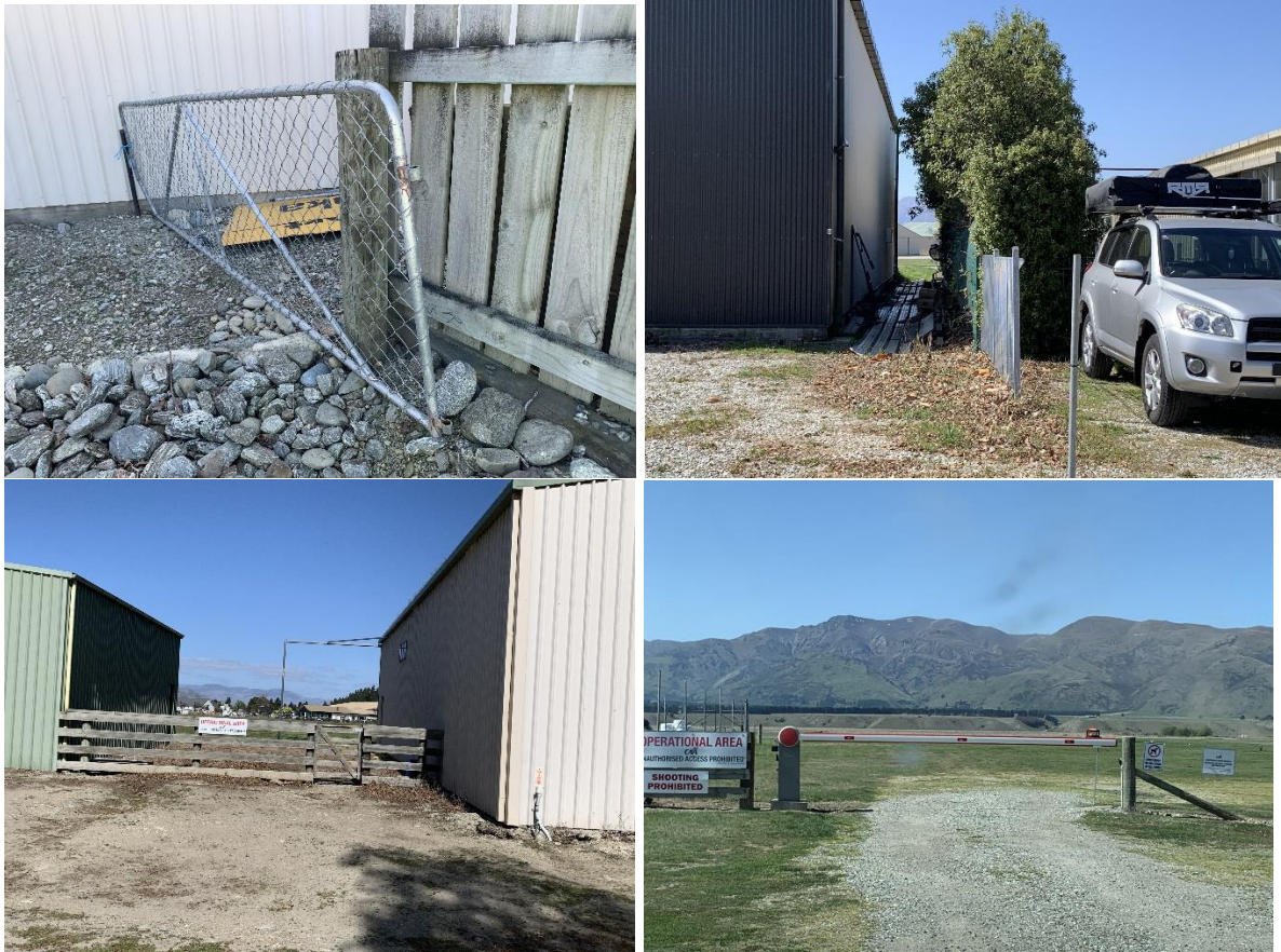
(clockwise from top left; unsecured gate, no fencing between hangars, inadequate fencing, barrier arm pedestrians and animals can get under or around)
