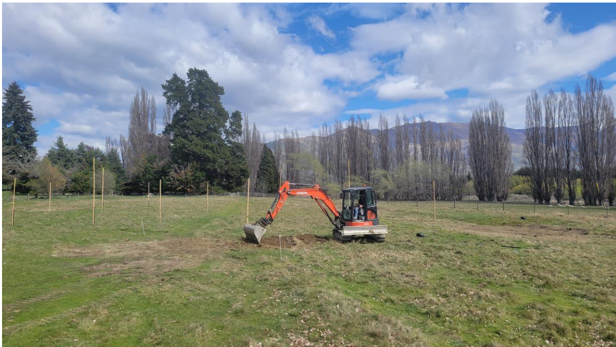
Photo 1 – Site photo taken during the investigations looking southwest over the proposed building platform location.
