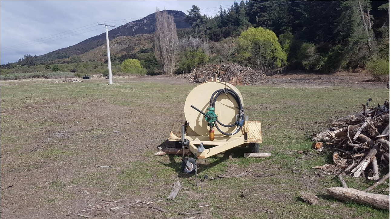
Plate 7: Portable diesel tank, appeared to be clean and in good repair.
