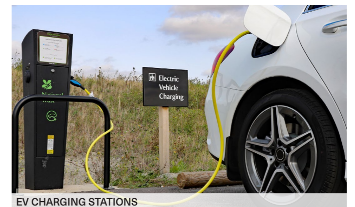
EV CHARGING STATIONS
