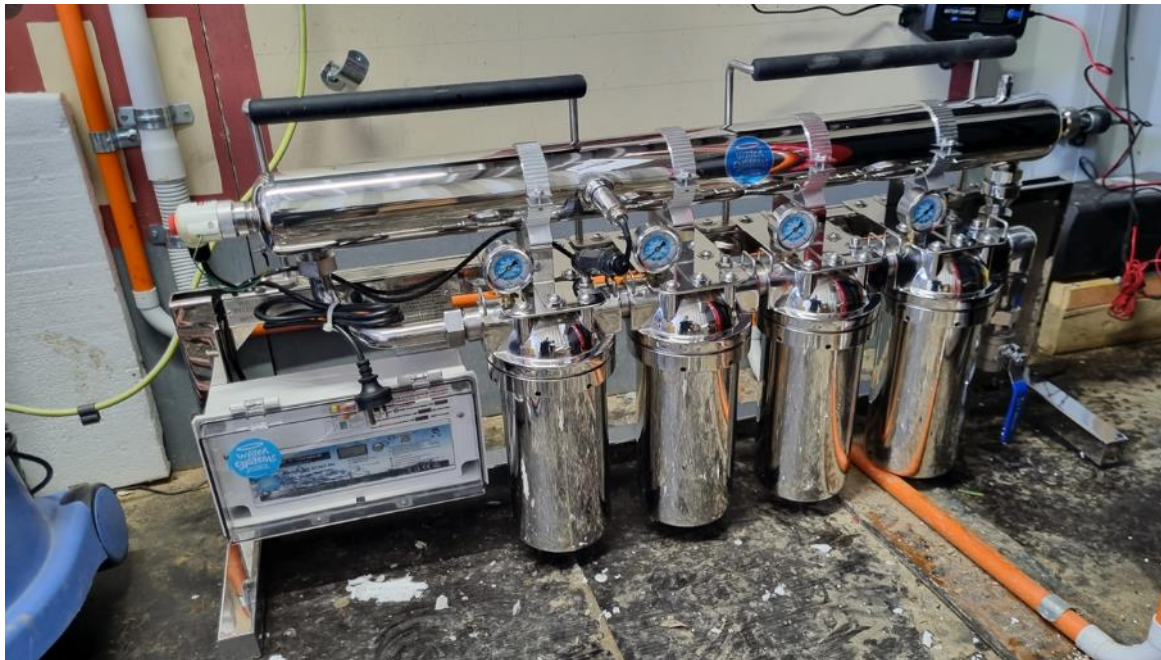
Snow Farm water treatment system prior to installation June 2024.
